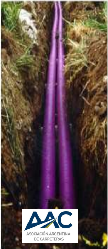
Ducts for cables
